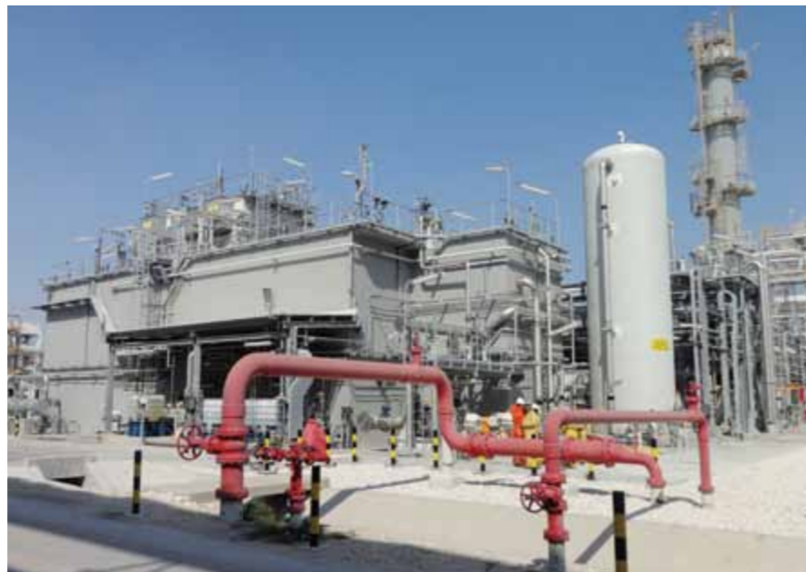
The completed Waste Water Treatment plant at Qatargas 1.
