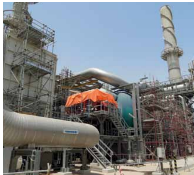
The recent shutdowns covered all the facilities of Qatargas 1 LNG Train-3, SRU-4, AGR-4, IR and part of Utilities Sea Water system.
